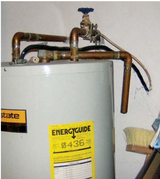
Photo: Discharge pipe too short. Photo by K. Hart.
