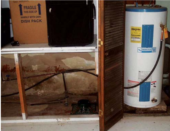
Photo: Constructed of old garden hose, a non-approved piping material, the discharge pipe on this garage located water heater was simply replaced with a run-off tube that terminated a couple of inches above the floor. Photo left K. Hart.
