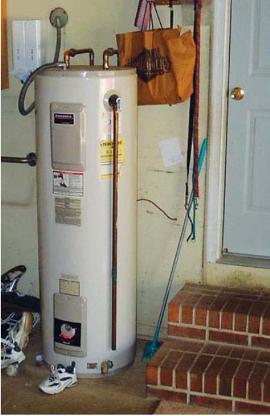
Photo: Water heater installed in a garage. Photo K Hart.
