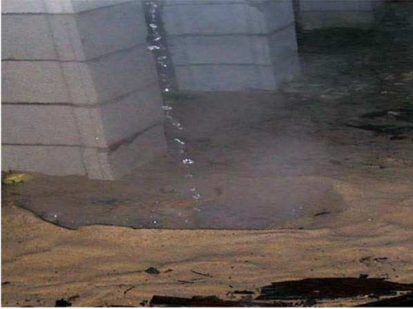
Photo: Discharging TPR valve in a crawl space. Photo by K. Hart.
