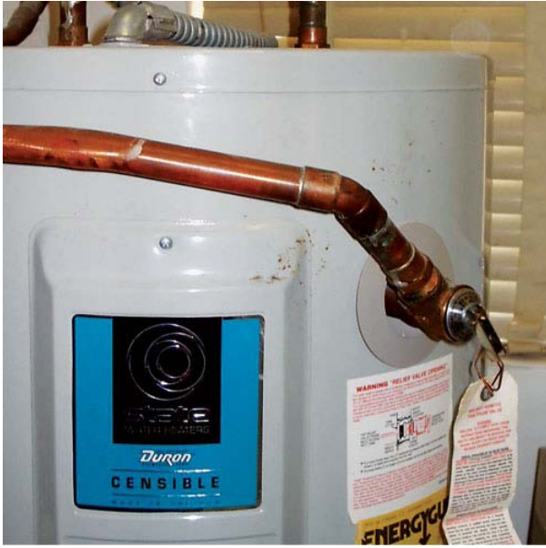
Photo: Trapped TPR valve. Photo by K. Hart.
